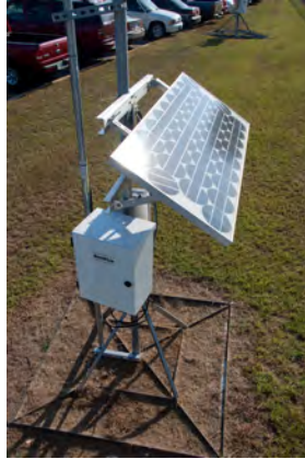
Figure 37 – Gateway Solar Panel
