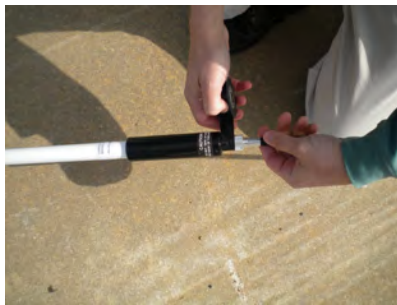
Figure 83 – Weatherizing RF Antenna
