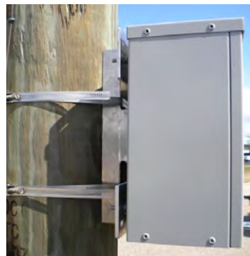
Figure 68 – UPS Attached with Clamps
