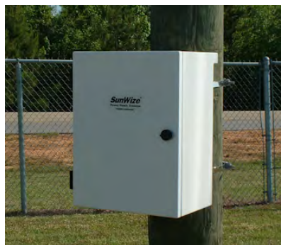
Figure 60 – Mounted Battery Box
