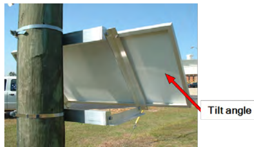
Figure 61 – Mounted Solar Panel
